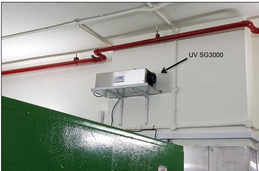
Raffles chose our UV SG3000T36 to remove odours in their bin centre
