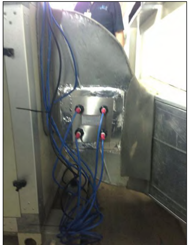
Right side of theatre 4 UV tube installation
