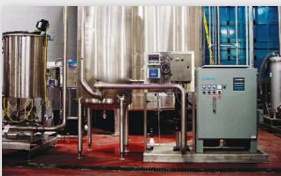
CD6000HO - Food Processing Facility
